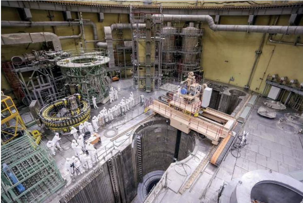
The reactor hall of the VVER-1200 (similar to the VVER-1000). The reactor vessel is pictured at bottom center. Photo: Rosatom
